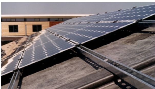
Figure 7.8 BP Solar system with visible mounting (diamonds). Langedijk-2 Meyersloot. □ Design BEAR-iD, Tjerk Reijenga.
