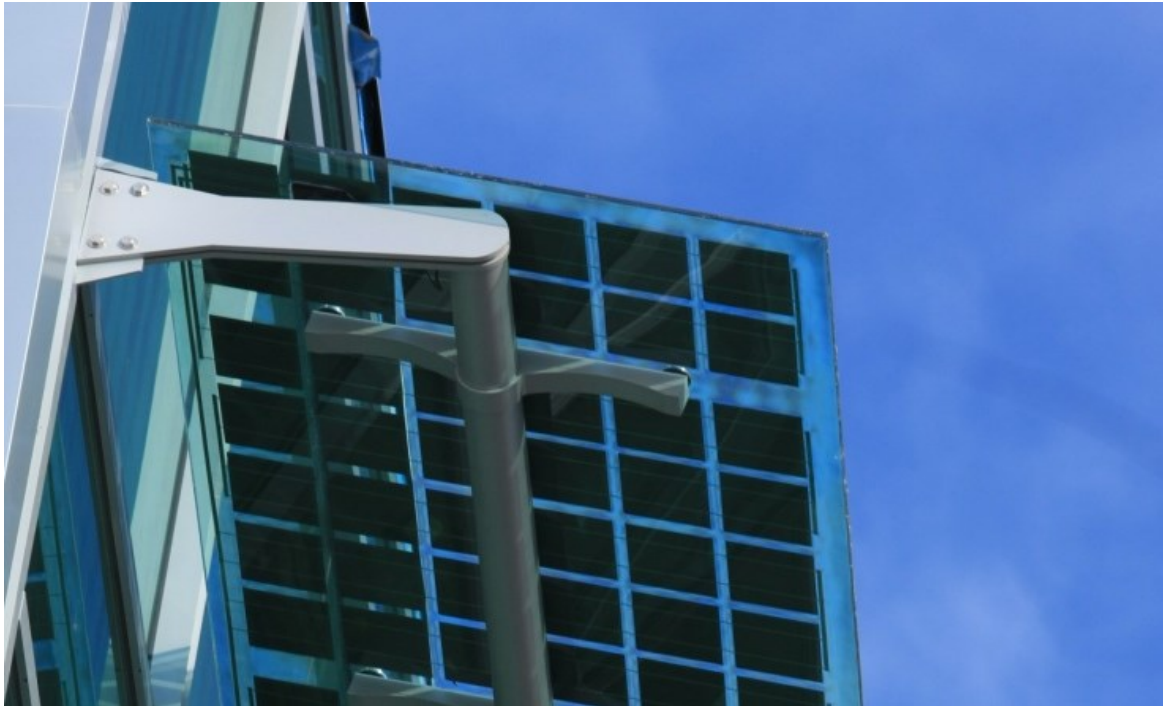
Figure 7.10 Fixings are more prominent than the actual lamella
