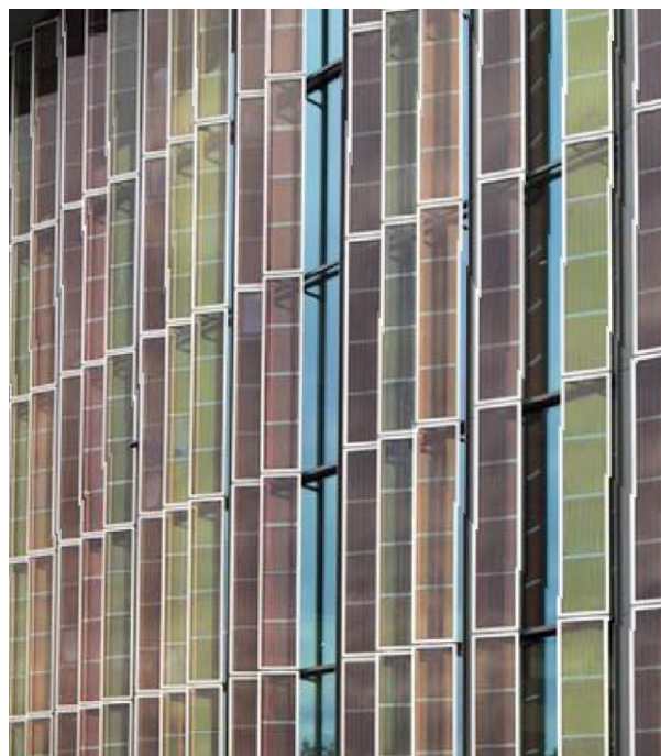
Figure 6.11 Vertical shading with Grätzel solar modules. SwissTech Convention Center, EPFL, Lausanne (CH). Photo: Hisashi Ishii
